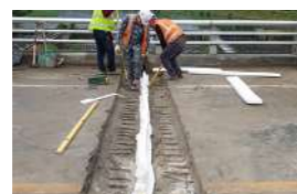
02. BLOCK OUT 철근노출
