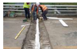
02. BLOCK OUT 철근노출
